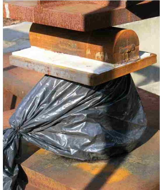
(b) Reaction Lebow-3129 covered by weather protection cover in bearing assembly
