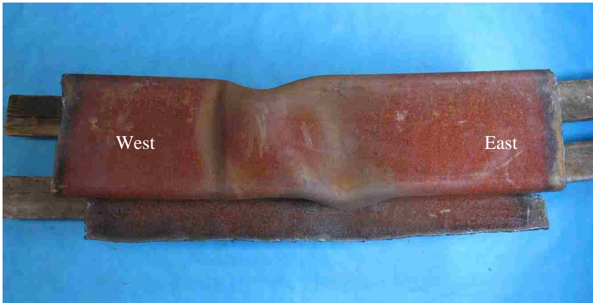
Figure 8.13 Buckled section looking from the inside of the curvature
