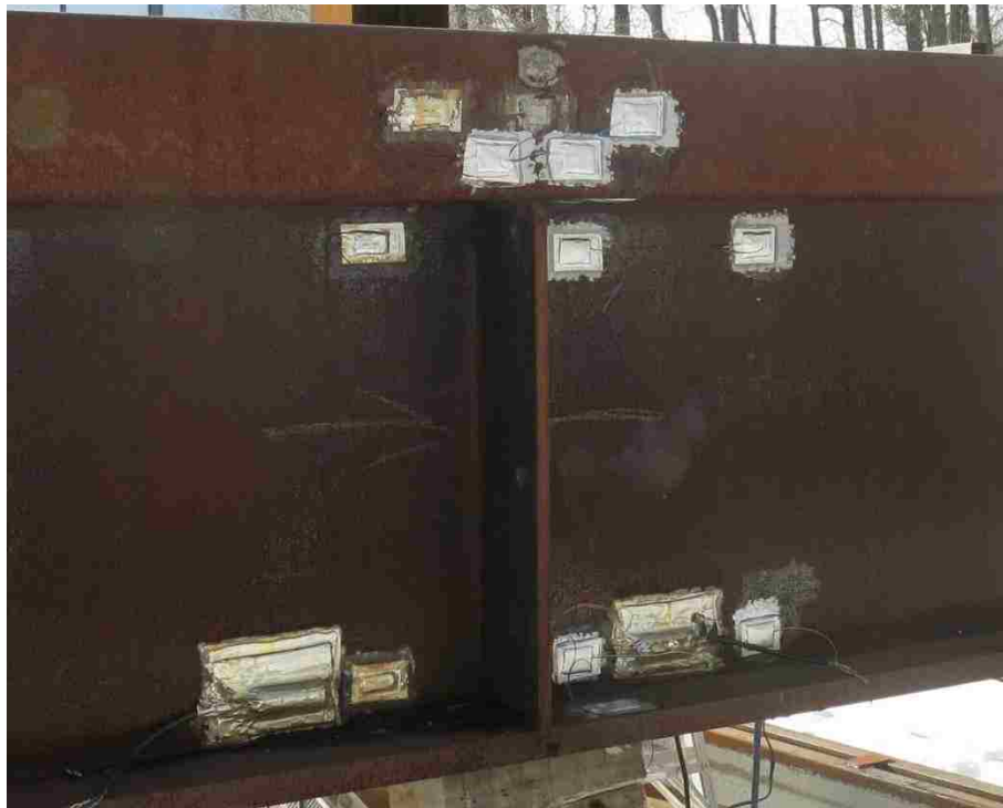
(c) Photograph of installed strain gages at Section G2_FM facing outside of curvature
